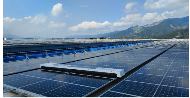
Tencent Data Center Roof Photovoltaic
